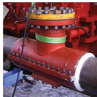
A 12" Grouted Tee fully installed
