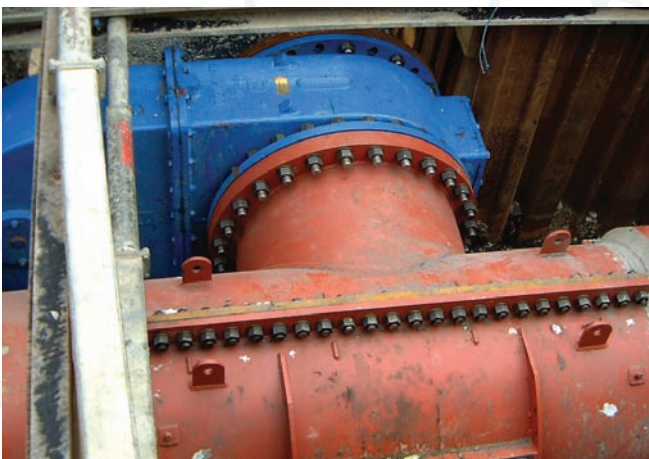
A 36" Grouted Tee fully installed
