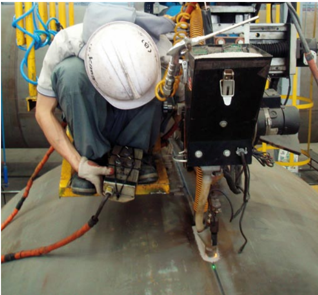
DIN 18800-7 – the key to jobs involving complex welding work, e.g. submerged arc welding of columns for wind turbines
