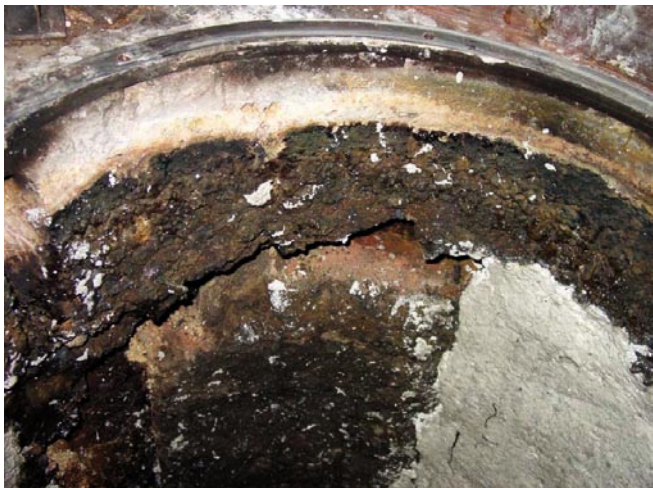
Damage caused by defect brickwork
