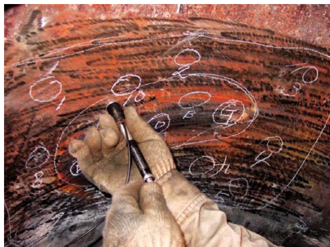
Hardness test to estimate extent of damage (damage survey)
