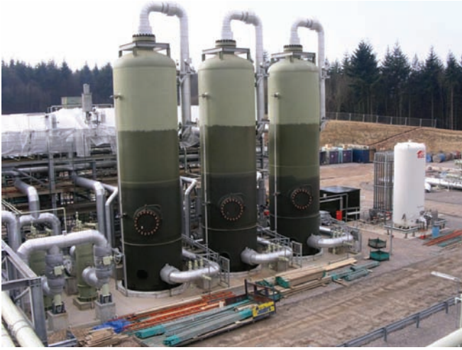
Figure 1: ADAPT Dewpoint Unit during the final stages of commissioning
