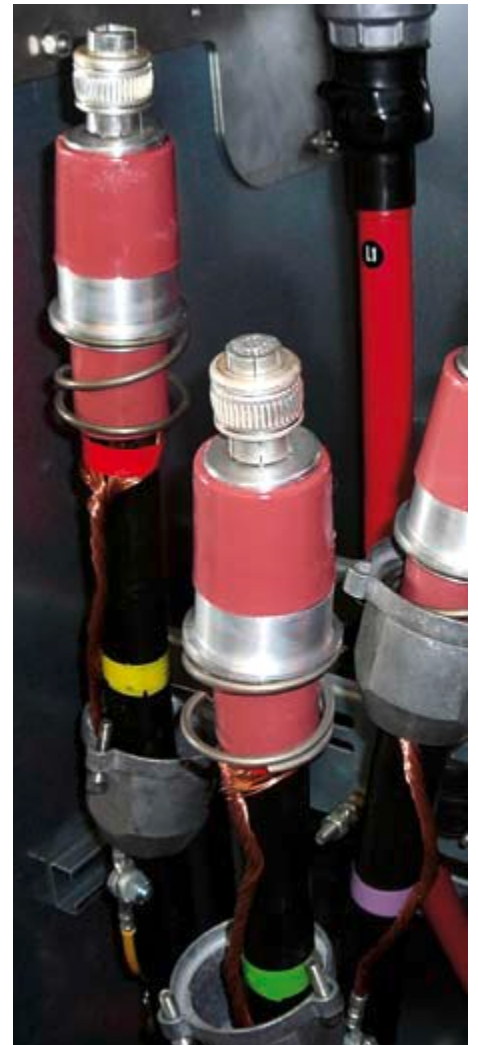
Medium voltage connection.
