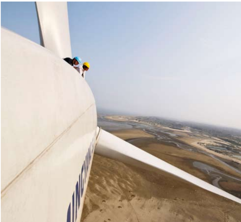
A prototype of Mingyang's 1.5-MW-turbine on the island of Xinliao Dao in the south of China.
